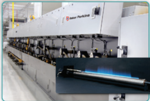
Direct Gas Fired Oven
